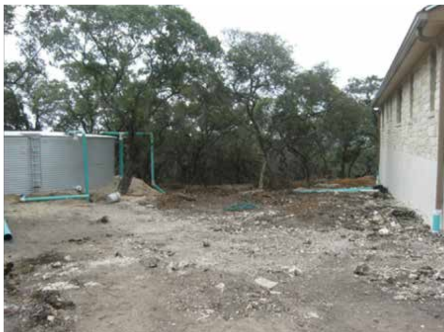
EARLY CONSTRUCTION OF the final tank and recapture system for a rainwater harvesting system.
